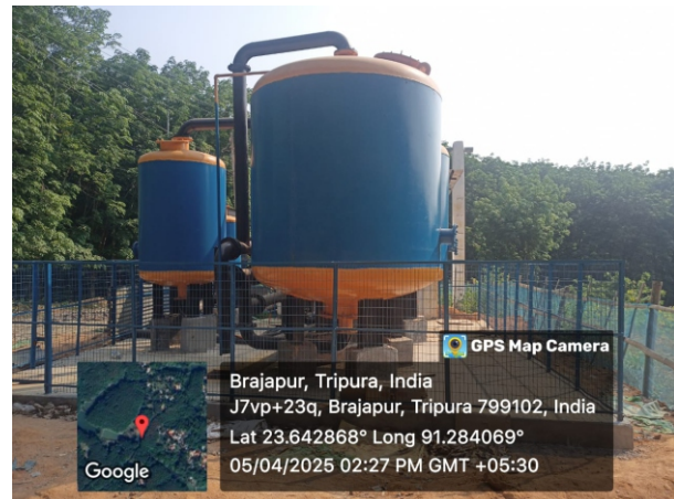
IRON REMOVAL PLANT
